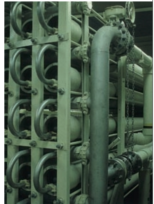
Pressure tubes that hold reverse osmosis membranes at a water reclamation plant.
