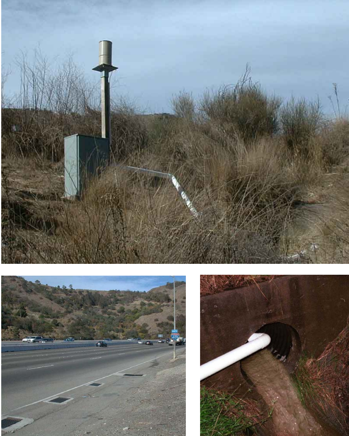
Figure 2.3 Pictures of Site 2, clockwise from the top: 1) site from a distance of 15 meters, showing rain gage, rain protection enclosure, PVC pipe for cables. The discharge is obscured by the brush; 2) drainage pipe showing free waterfall and PVC pipe for cables for level and velocity sensors, and 3) freeway looking north showing the four inlet grates.
